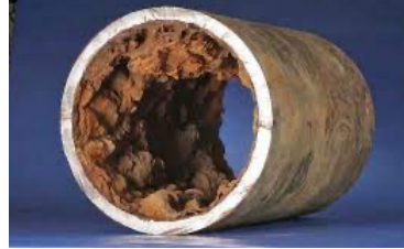
Tuberculation in Pipe
